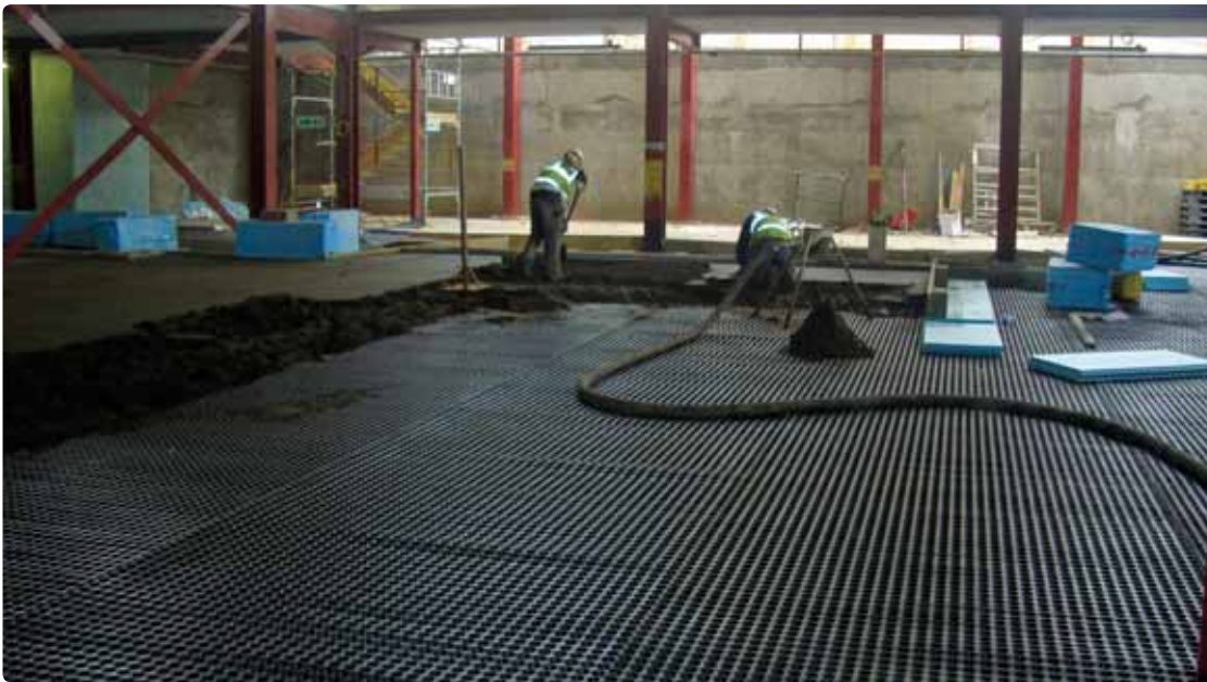
Figures 2-3: Installation of a watertight concrete system to walls and floor, including Platon P20 (Figure 2).
